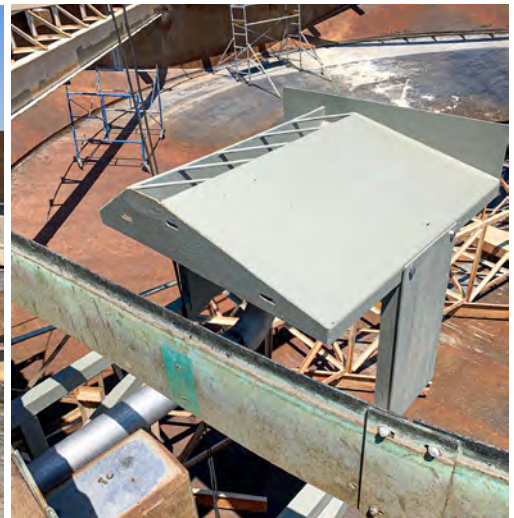
New scum box installed on Primary Clarifier #4
