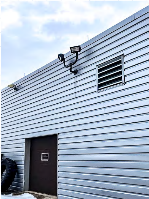
Exterior security lighting at the Sheboygan Police Department
