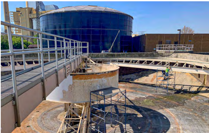
Touch up painting in Final Clarifier #2, showing corrosion on the stilling well
